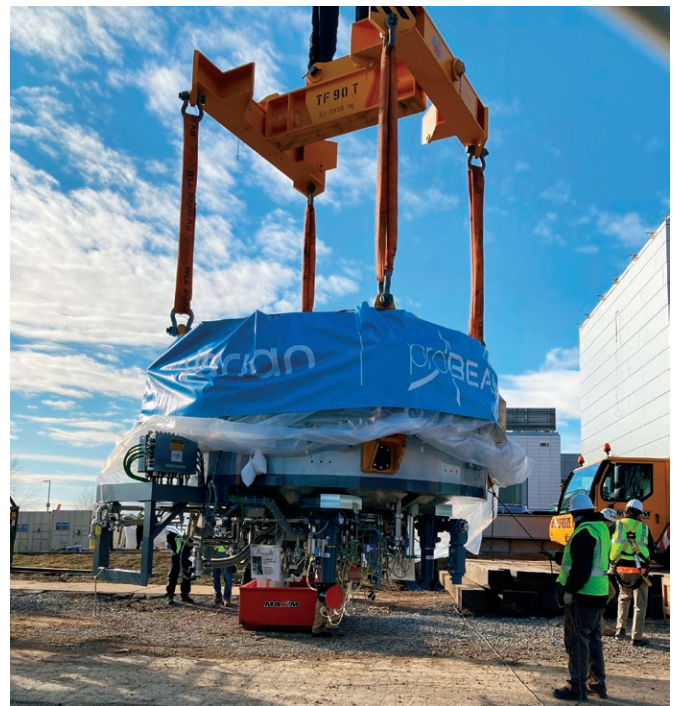
The $48 million proton therapy project at LGH hit a milestone in January. The cyclotron, a centerpiece of the technology weighing as much as a 747 airliner, was delivered via tractor-trailer and hoisted and lowered into its new home.
